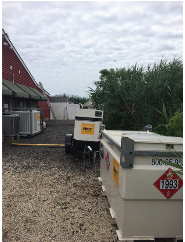
In the photo: Industrial air conditioners and a generator that Herc Rentals installed at an Ocean City, N.J. animal shelter on a temporary basis this past July after an equipment breakdown.
